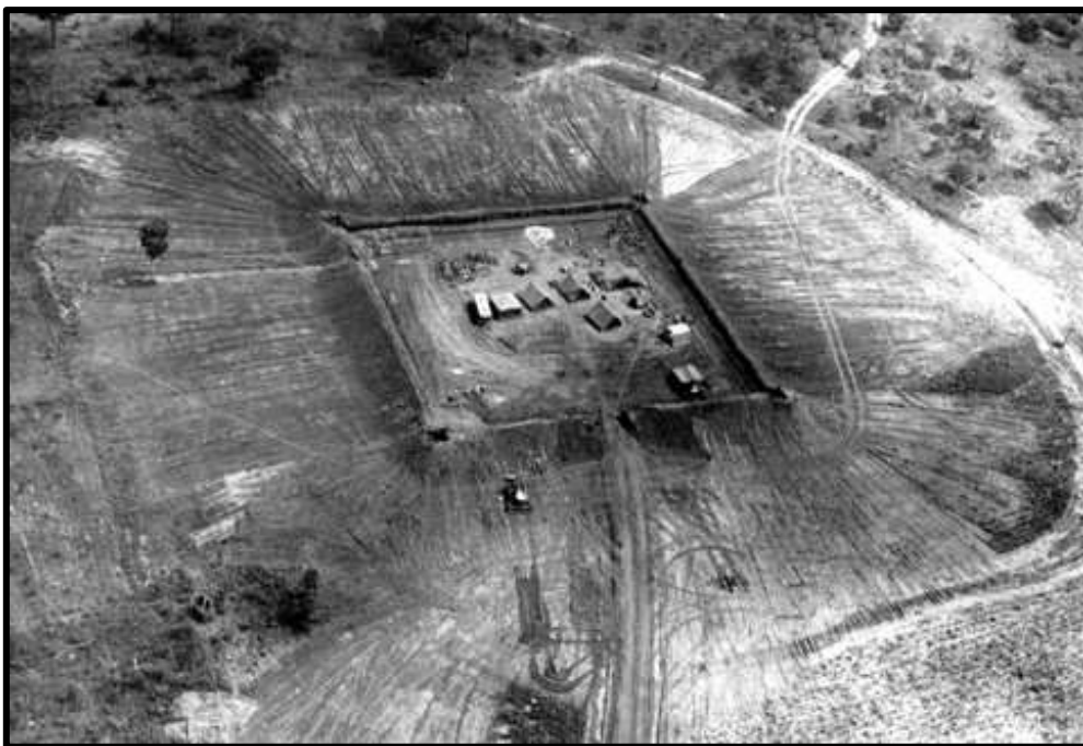
Graphic image of a Bulldozer forming the earthen walls of a keep (Ft Misery, Nembire, Mt Darwin) (Gerry van Tonder collection)
